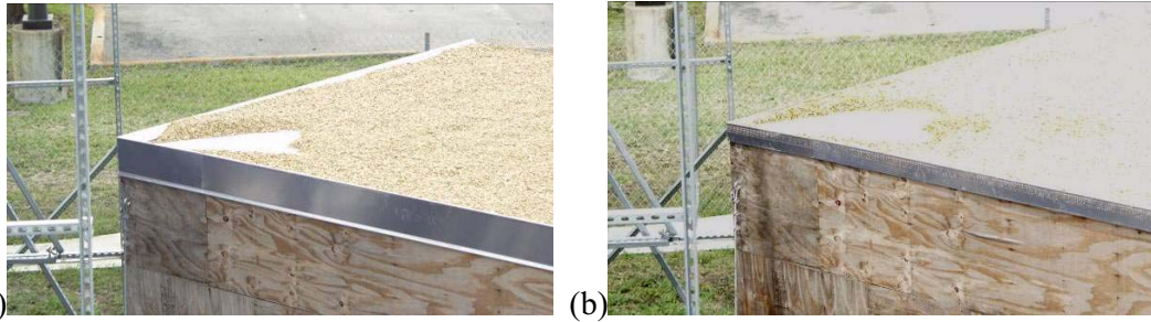
Fig. 9. Gravel scour recorded for conventional products at a wind speed of 74 mph (38 m/s) for a cornering wind of 45°: (a) Traditional fascia; (b) Drain-through gravel stop
