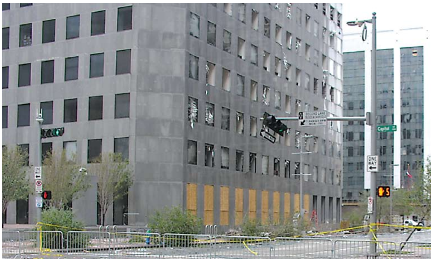
Figure 9: Commercial window cladding damage was limited to a few sporadic cases.
