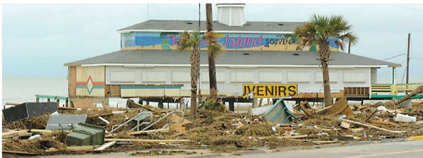
Figure 13: Galveston Island beach-front commercial buildings. Storm surge was significant, as evidenced by the debris line. However, the roof cover has minimal damage, indicating winds speeds were lower than expected.
