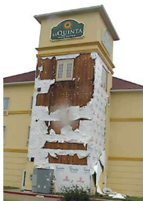
Figure 8: Cladding that employs Exterior Insulation and Finish Systems (EIFS) were particularly vulnerable to failure.
