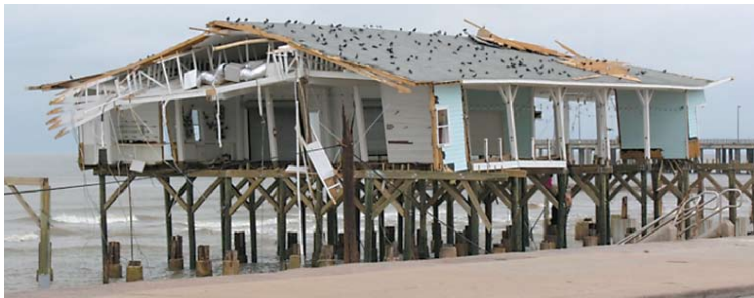
Figure 12: The beach at Galveston Island. Storm surge was significant. Note that the roof cover has minimal damage, indicating winds speeds were lower than expected.
